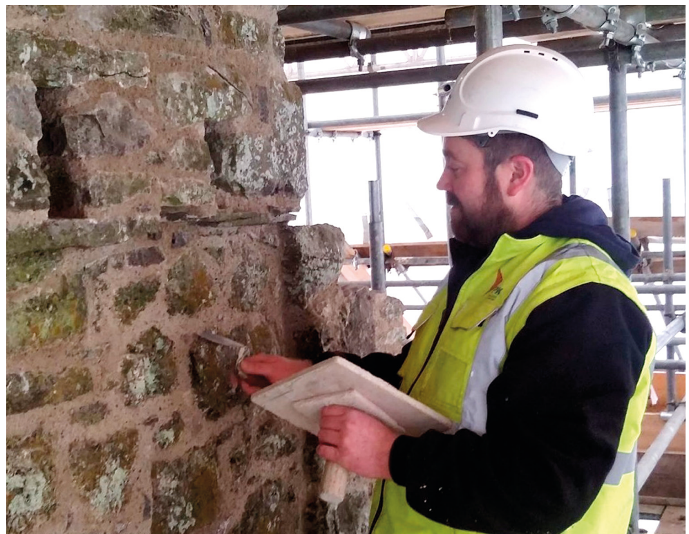
Conor O'Brien, apprentice stonecutter/stonemason working on conservation of the gate tower at Kells Priory, Co. Kilkenny
